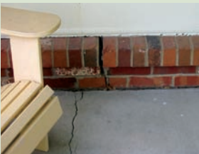
Mine subsidence can cause cracks in pavement or foundations, as shown above.
