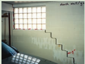
Step cracks, such as these, are not uncommon in block walls affected by mine subsidence.
